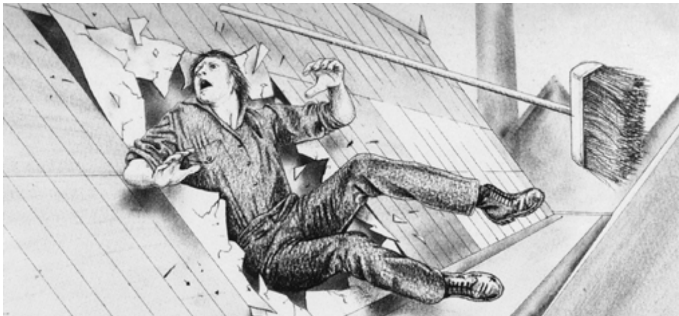
A man cleaning valley gutters on an asbestos cement sheet roof stumbled and fell to his death
