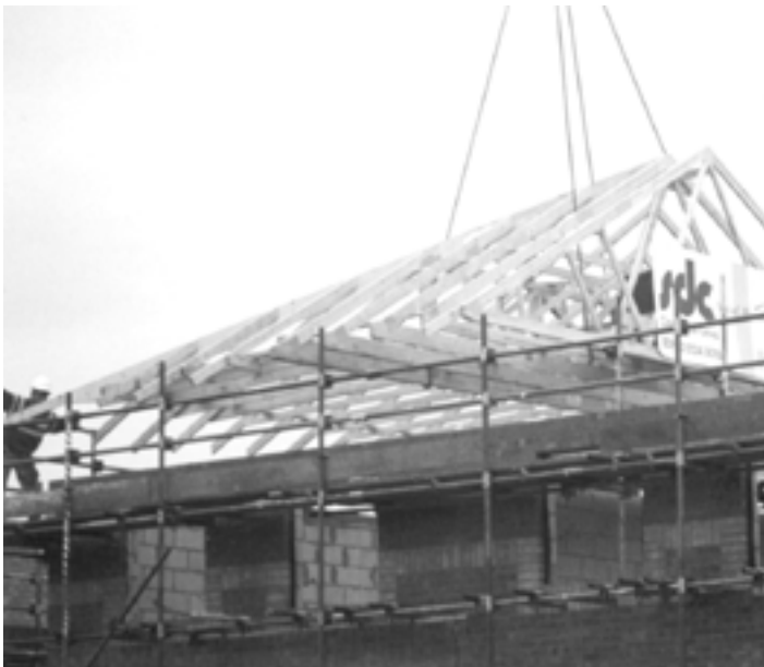
Roof truss built on ground and lifted into position avoiding the need to work over open joisting later on
