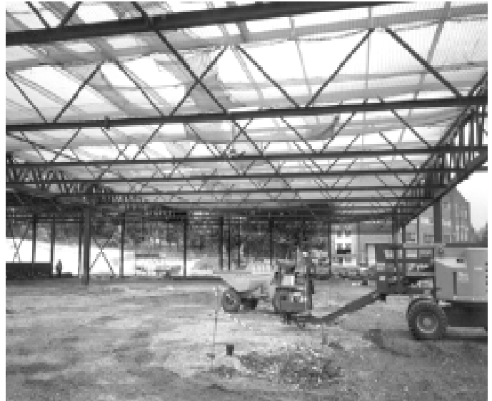
Safety nets installed prior to sheeting. Note the net is fixed as close to the underside of the roof as possible to minimise the extent of any fall
